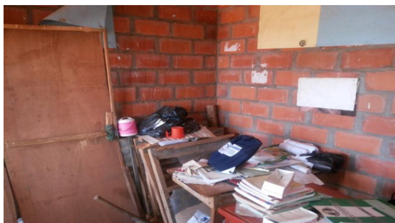
Plate 5: Classroom used as Store at LGEA Primary School, Danhonu, Chikun LGA Source: Fieldwork (2018)
